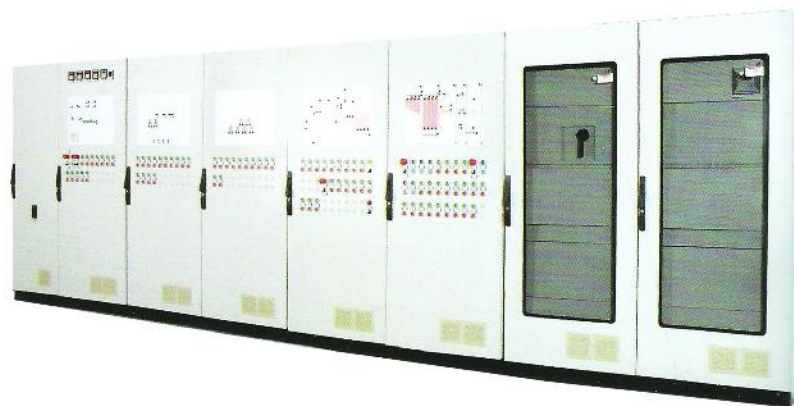
MCC Command Control Panel
