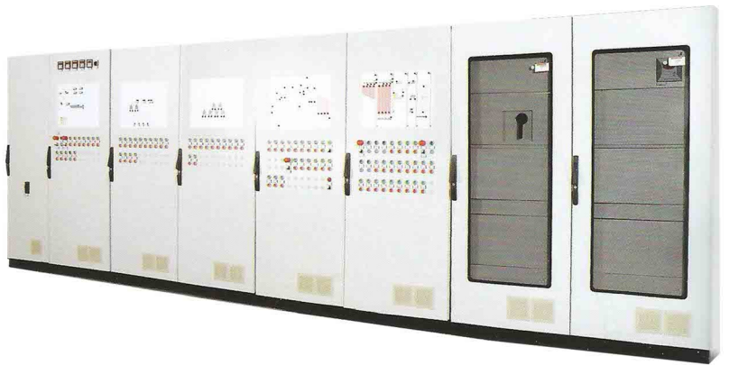
MCC Command Control Panel
